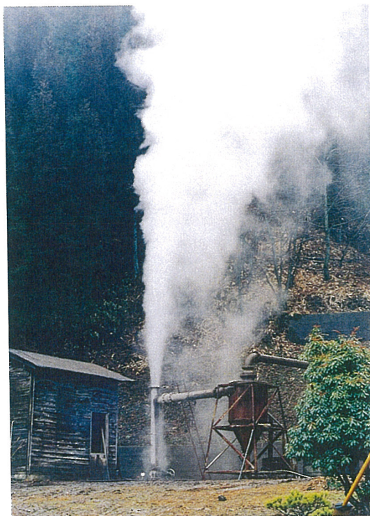
飯田観測所の噴気井 Steam well at Handa Station
